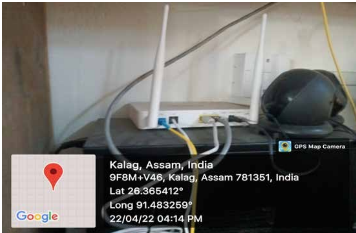
BSNL Fiber Wi-Fi internet connection
