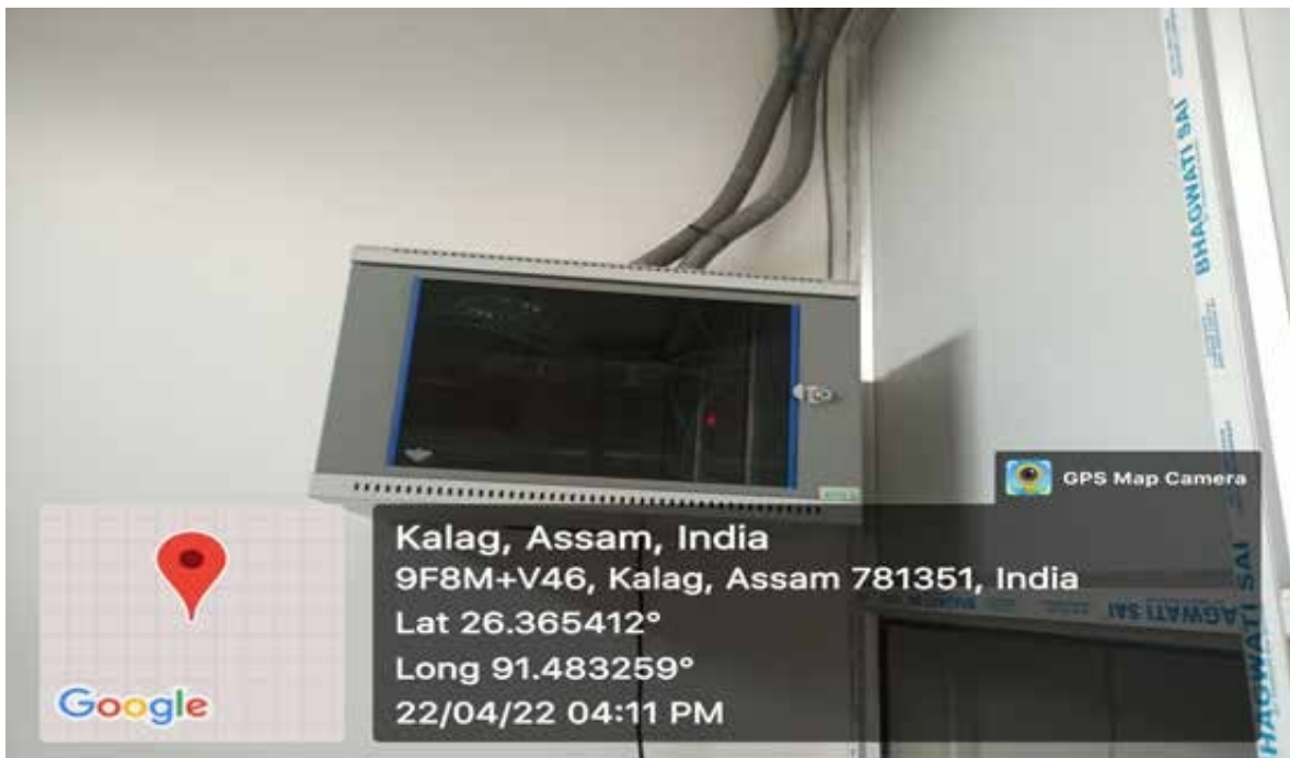
LAN Gigabyte Ethernet switch
